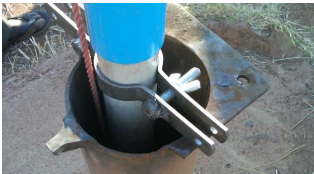
(a) Broken flanges on Afridev pump in Malawi Source: Larry Bentley.
