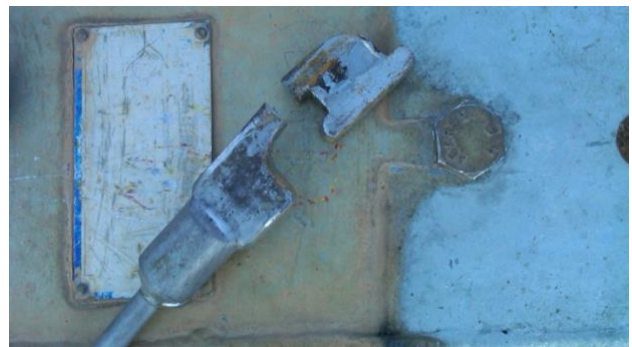
(b) Broken hook on Afridev pump in Malawi Source: Larry Bentley.
